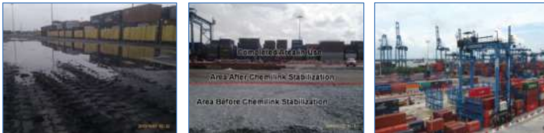
a) Before Upgrading b) Before and after Stabilization c) Upgraded Yard in Operations
