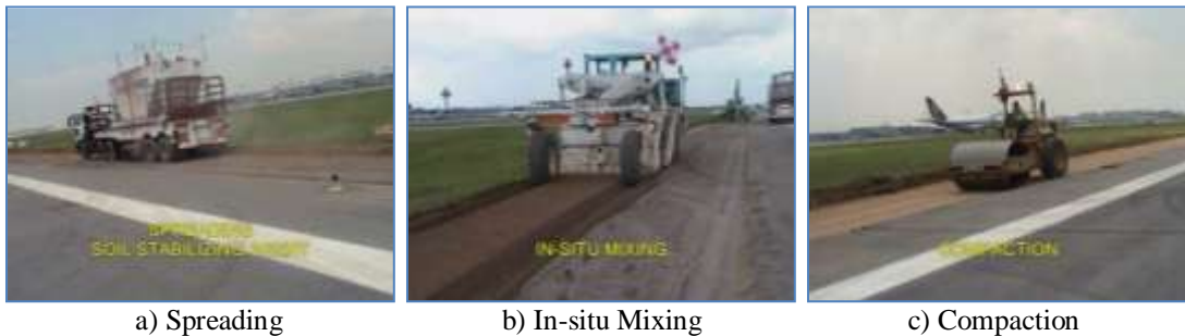
Photo. 1. Typical In-Situ Mixing Process of Soil Stabilization (Photos source: Singapore Changi Airport Runway Widening)
